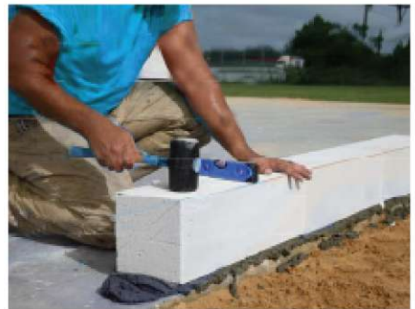
Figure 5D.4: Checking level and plumb, modify by tapping VODAPRUF ALC Block with rubber mallet
